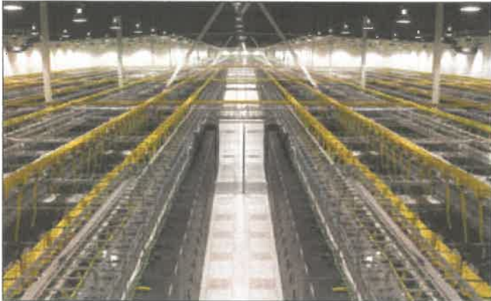
Mission operates its SCADA service from a carrier grade computer co-location center located near Atlanta, Georgia.
